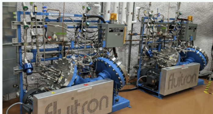
Circulation compressors (gas)
